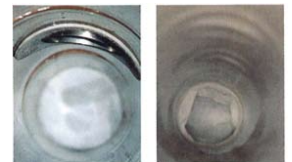
Lateral pipes are inspected using the National Liner robot with CCTV cameras to determine liner specifications.
