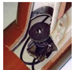
The S collar protects lateral pipe entrances
