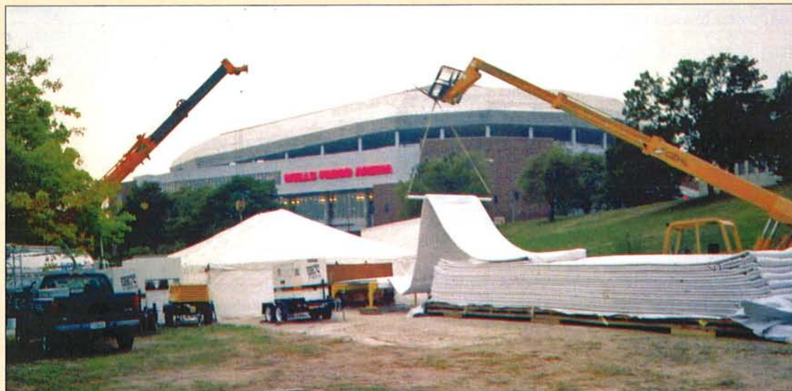
Large diameter felt tubing was readied for wet-out near the busy Wells Fargo Arena.
